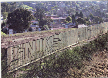
Graffiti vandals have taken the opportunity to showcase their "tags" on the back fence of a new housing development.
